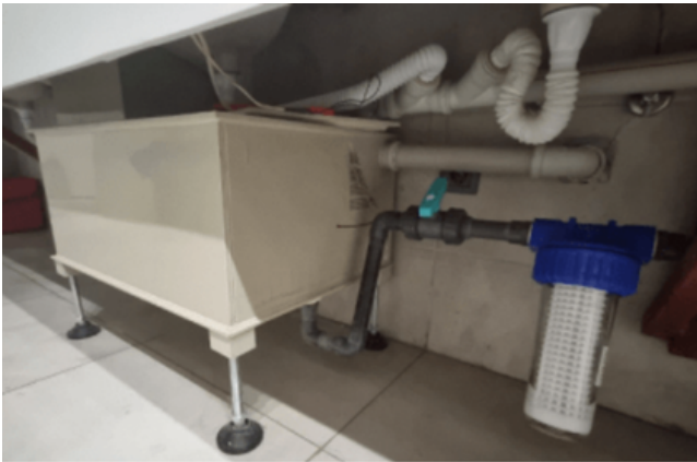
IMU Greywater Recovery System
